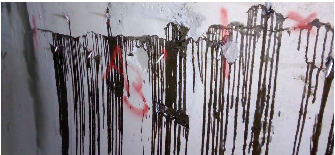
CONCRETE CRACKS REPAIRS
